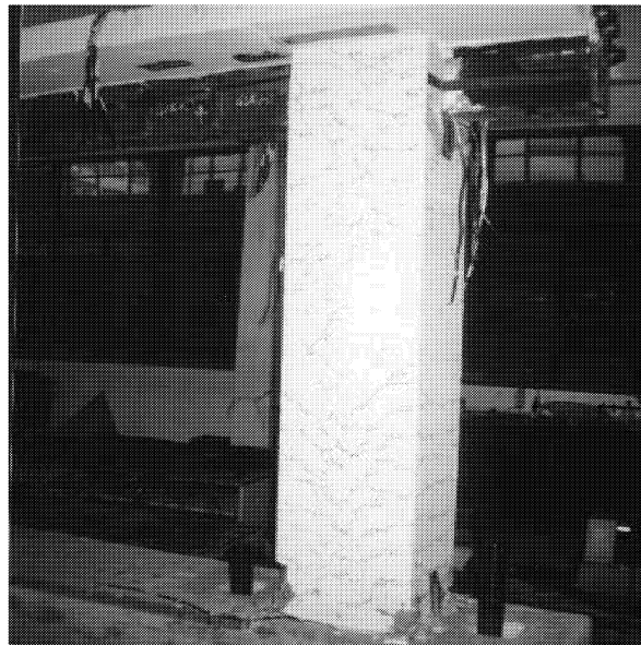
Figure 6. Failure of frame columns
