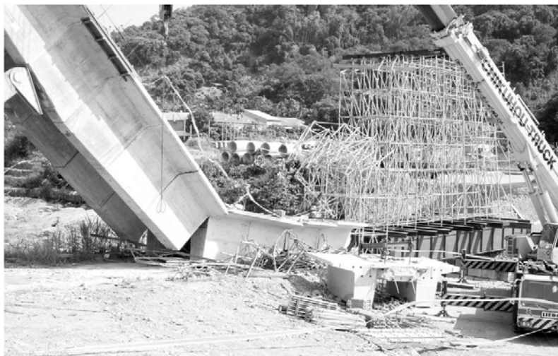
Figure 1. Scaffold Collapse Occurred at a Construction Site in Taichung, Taiwan [1]
