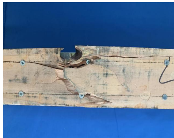
(d) Further destruction of the planks between the self-tapping screws along the smooth grain observed at the web of the L-5 beams
