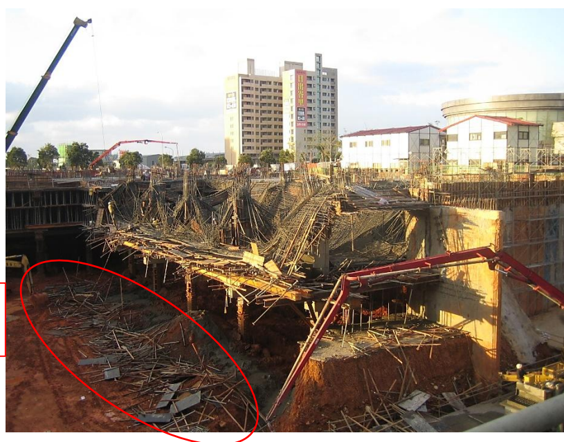
Fig. 5 Collapse of double-story temporary support at the Linkou residential project in Taipei, Taiwan
