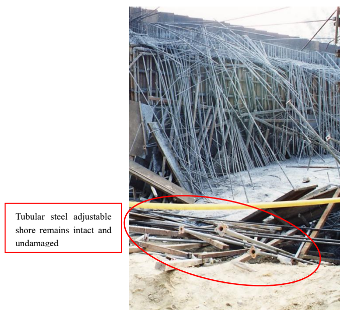
Fig. 4 Collapse of single-story temporary support at the box culvert on Second Expressway in Kaohsiung, Taiwan
