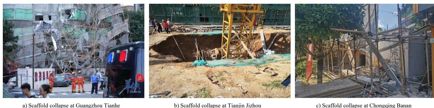
Fig. 2 Engineering accidents caused by scaffold collapse
