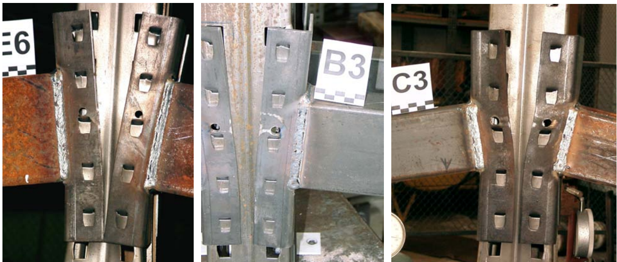
Figure 22. Typical Deformation of Internal Joints Observed in Each Joint Group
