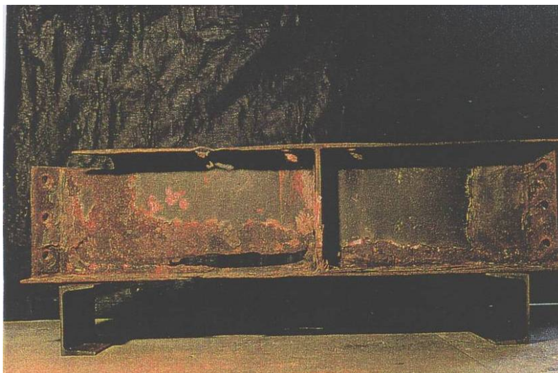
Figure 1. The Identical Corroded Universal Steel I-Beams
